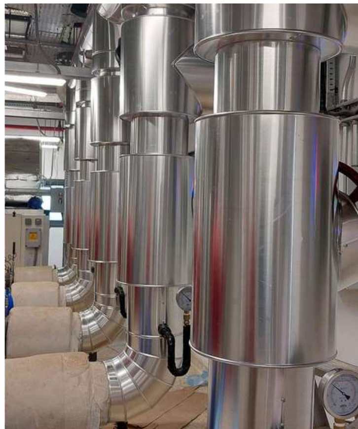
Pumping Station of Chilled Water for Air- Conditioning Systems
