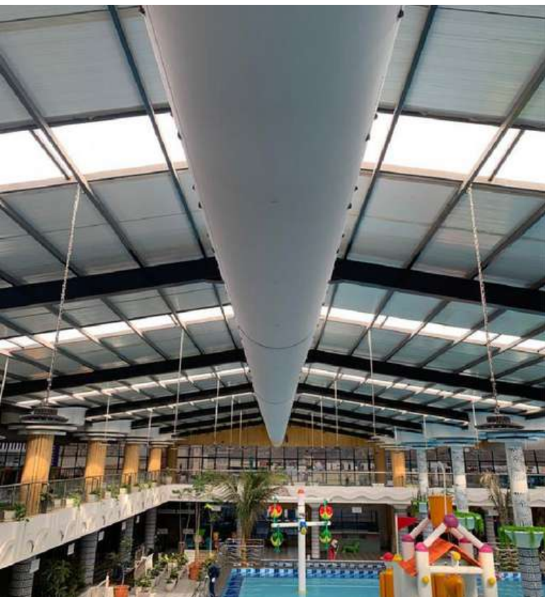
Mechanical Engineering Department Mega space MEP Work
